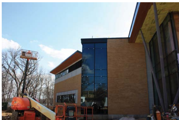
Edgewood College's Visual & Theatre Arts Center, seen here under construction, will be open for the Fall 2012 semester.
