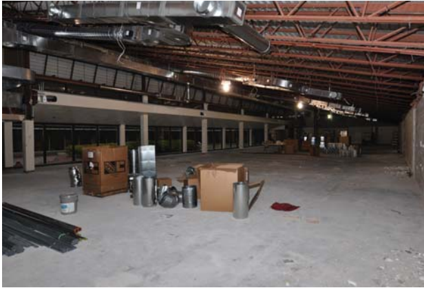
A former telephone call center is being converted into the new Carroll University Graduate Center that will open this fall.
