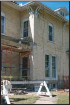
A construction worker rehabs a side porch at what is to become Ripon College's Evans Welcome Center.
